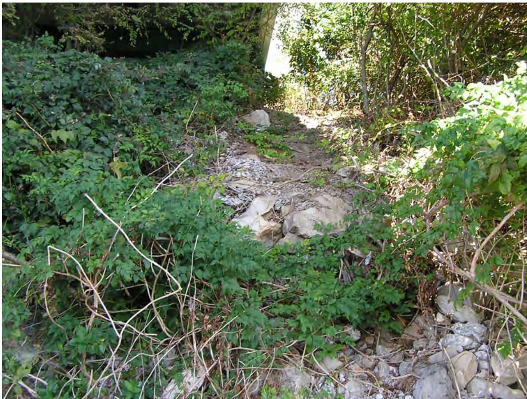
Photo 10: View facing north from north bank under SR-92 bridge over French Broad River.
